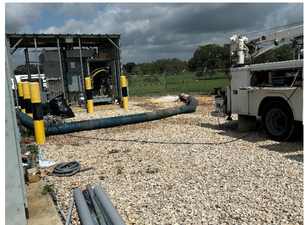
Well 14 – Pump Start up
